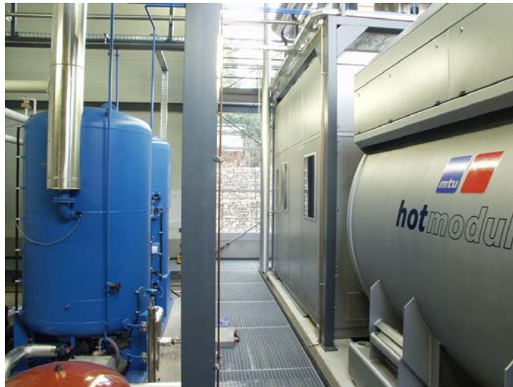
Figure 5: HotModul – Multi Effect absorption chiller combination in Bad Berka, Germany
