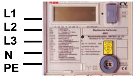
Four quadrant meter
